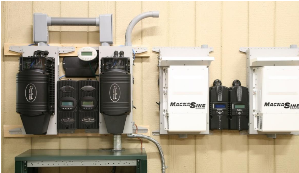
OutBack and Magnum horizontal stacked systems
