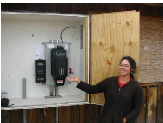
A Positive Energy installation, NM
