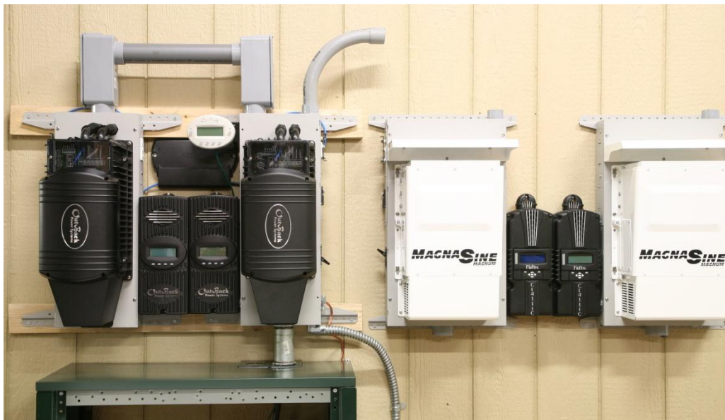
OutBack and Magnum horizontal stacked systems
