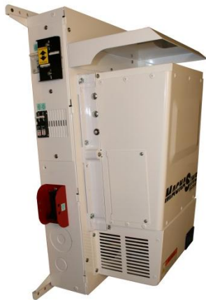
Left Hand Magnum as installed
