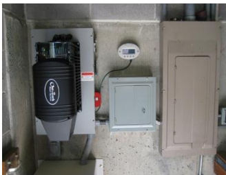
A Jay Peltz installation, CA In the basement
